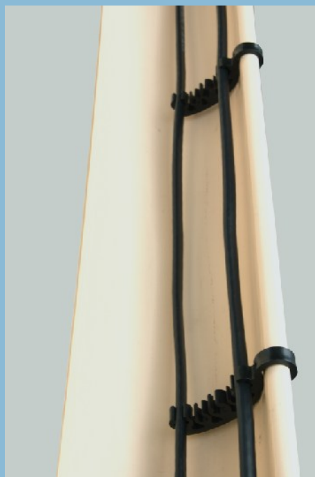
Heating cables installed in a gutter using the clips
